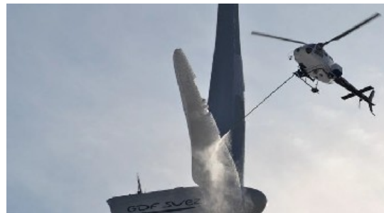
Deicing wind turbine blades
